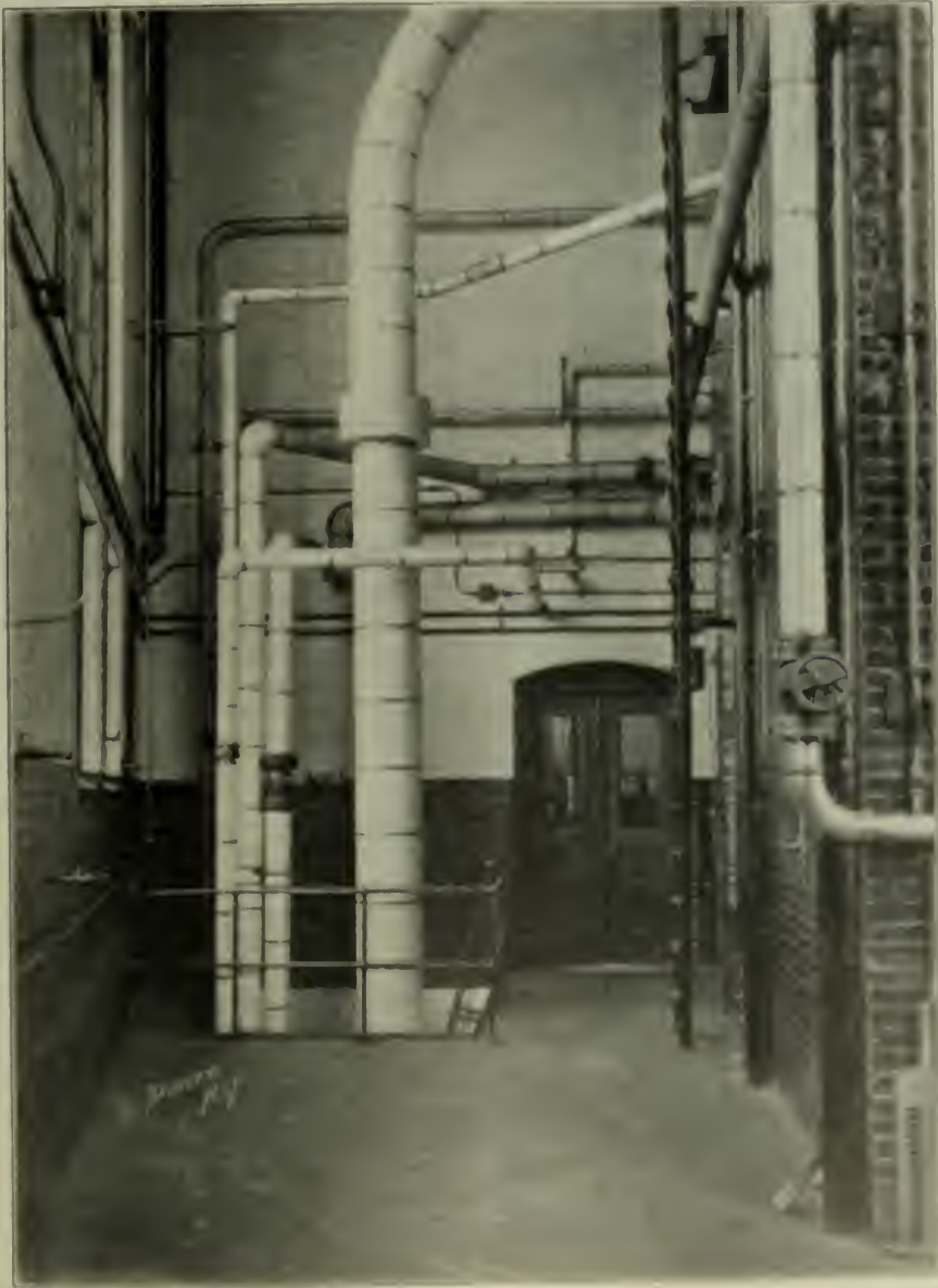
FIG. 3. STEAM ROOM EQUIPMENT, TURBINE.
